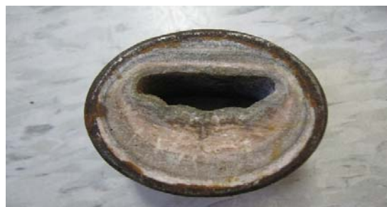
Figure 1 Scale of Boiler
