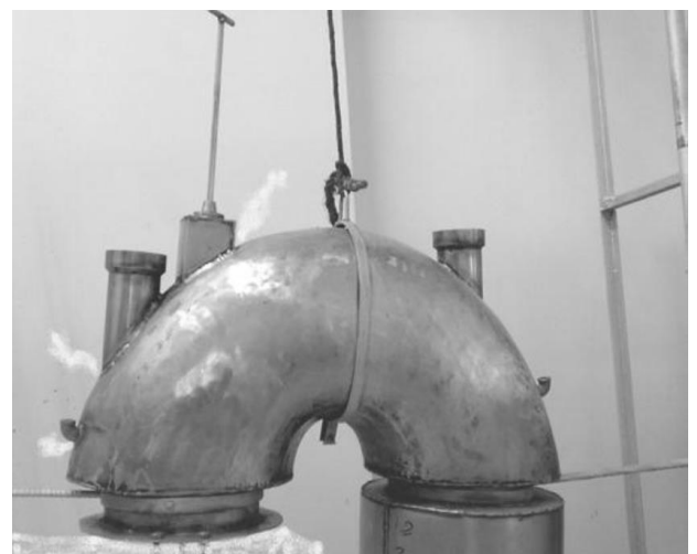
Figure 2 shows smoke evolving from areas of vacuum leaks
